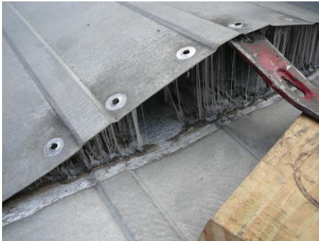
BUTYL SEALANT WEBBING BETWEEN ROOF PANELS.
