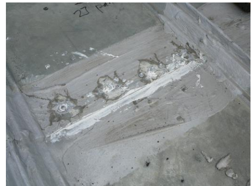
RESEALED ROOF PANEL END LAP JOINT.
