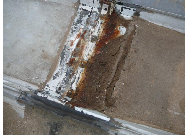
REMOVED EPDM MEMBRANE REVEALS SEVERE CORROSION.
