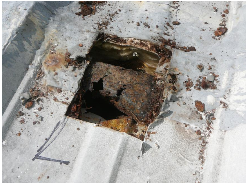
SEVERLY CORRODED ROOF PURLIN UNDER RUSTED ROOF PANEL.
