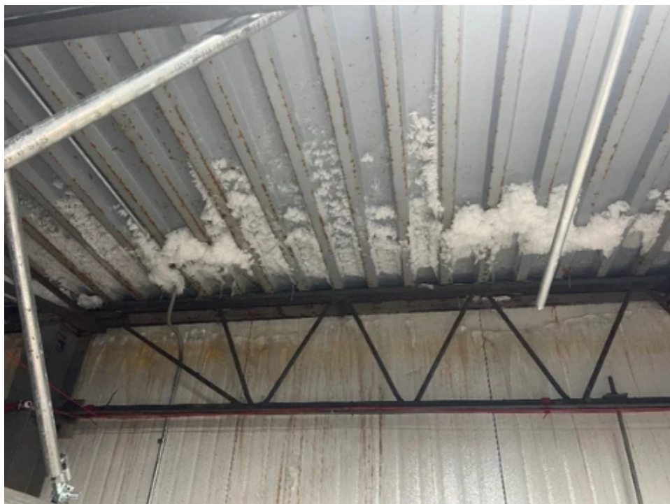
Ice accumulation at a roof-deck-to-wall transition — a signature of condensation caused by air infiltration.
