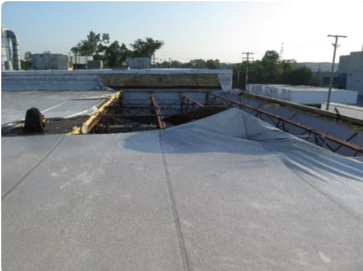
Roof blow-off caused by severe deterioration of steel decking along a brick parapet wall — the end state of unmanaged, cyclical condensation.
