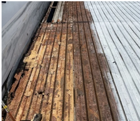
Steel roof decking corroded through by prolonged, unmanaged condensation exposure.
